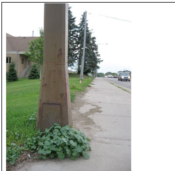
Rusted streetlights in Mound that will be replaced with stimulus dollars. June 2009.
